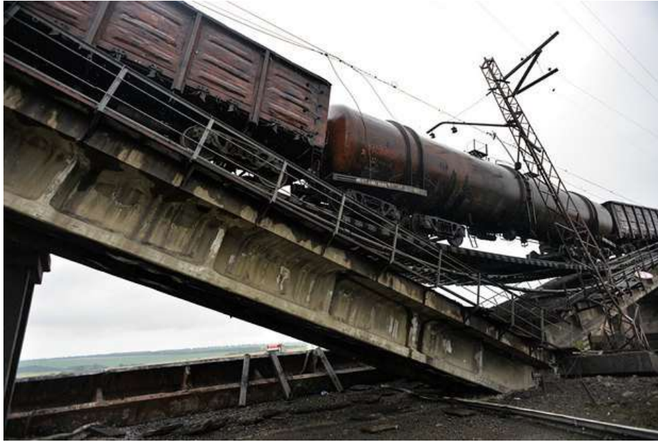
Fig. 4. Destroyed railway bridge.
